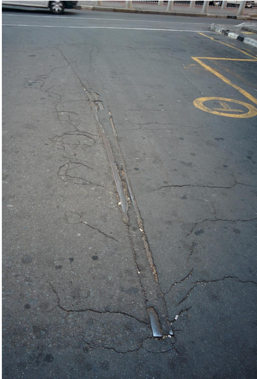
Figure 34. Old tram railways coming out of the tarmac after years of wear.
