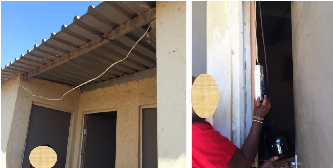
Figure 5 Seen above is the hazardous electricity connection and wiring extended from the main house ©Hopa, Zola, 2016
