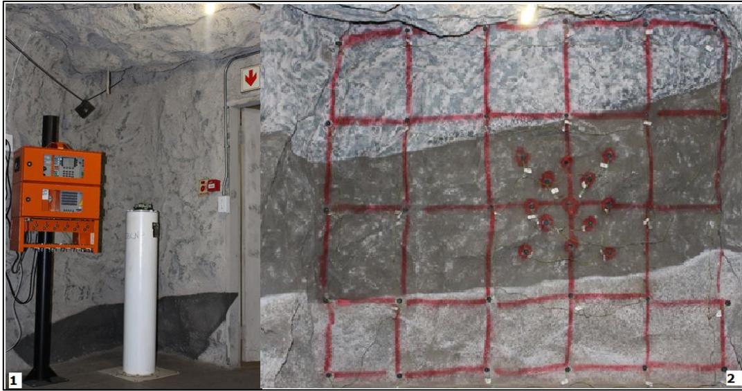
Figure 5.2 (1) DetNet Blasting Unit (2) Timed Development End Face
