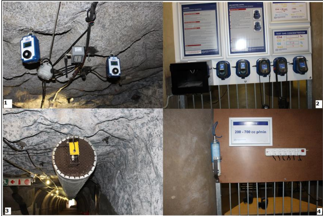
Figure 5.9 Mine Ventilation Systems installed in the Wits DigiMine Mock mine (1) Fixed Gas Detectors (2) Sentinel Handheld GDI (3) Velocity Meter on an ventilation duct (4) Methane Calibration Gas Canister
