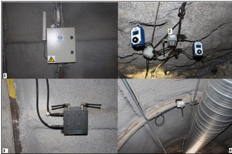
Figure 5.3 (1) Schauenburg MIMACS Communication device (2) Fixed gas detectors & Minetec tracking Node (3& 4) Minetec tracking Nodes and ventilation duct
