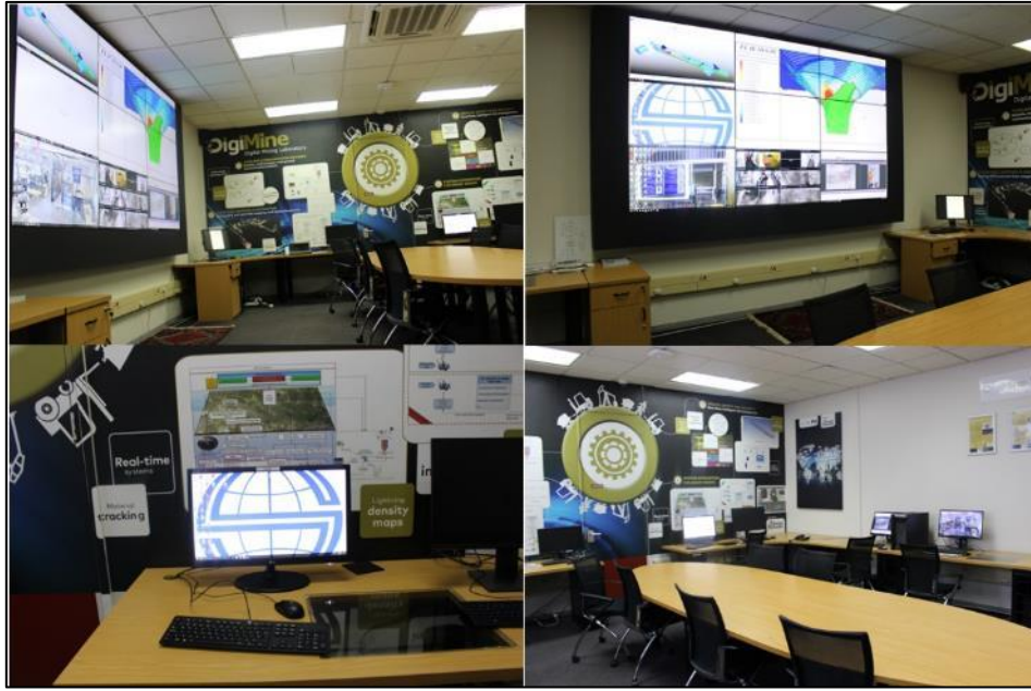
Figure 5.4 Overview of the Wits DigiMine Control Room
