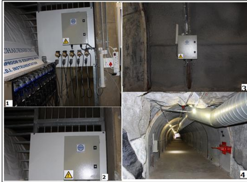
Figure 5.8 showing the Schauenburg Lamproom S-link (1and 2) and Tunnel S-link (3 and 4)
