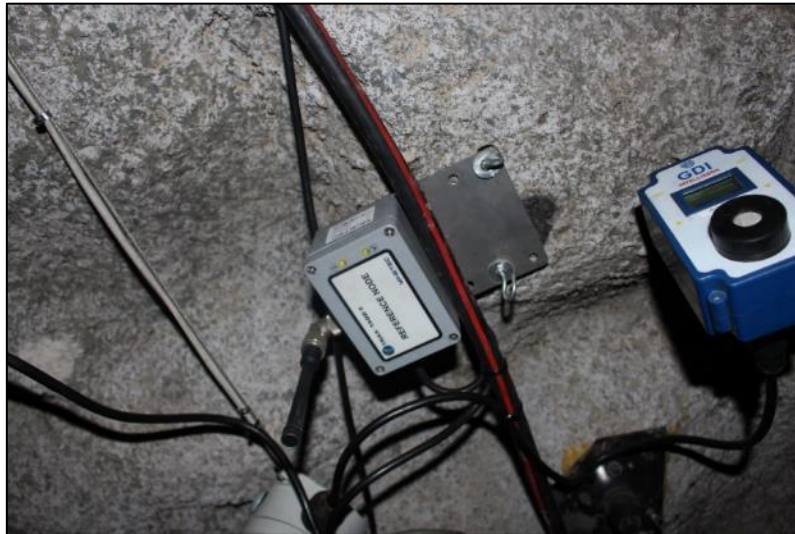
Figure 5.16 Minetec Reference Node mounted in the Mock Mine Tunnel Roof
