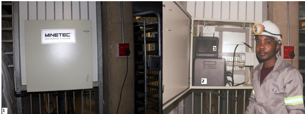
Figure 5.19 Minetec box (1) housing an Uninterrupted Power Supply (UPS) (2) and Rugged In-vehicle-PC (3)
