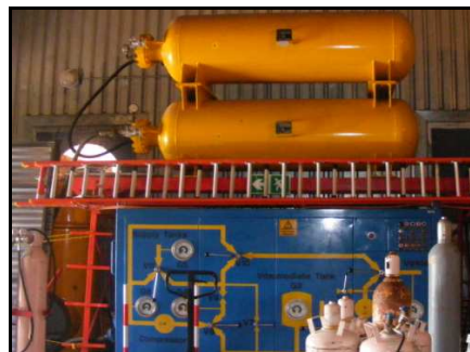
Figure 10: Gas compressor and vacuum pump fitted with storage tanks
