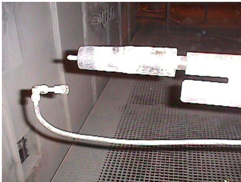
Figure C.5: The slag probe without the removable slag sleeve. The tapered front end is evident. The aluminium tube supplying cooling water to the slag probe is in the foreground. The boiler wall is on the lefthand side.
