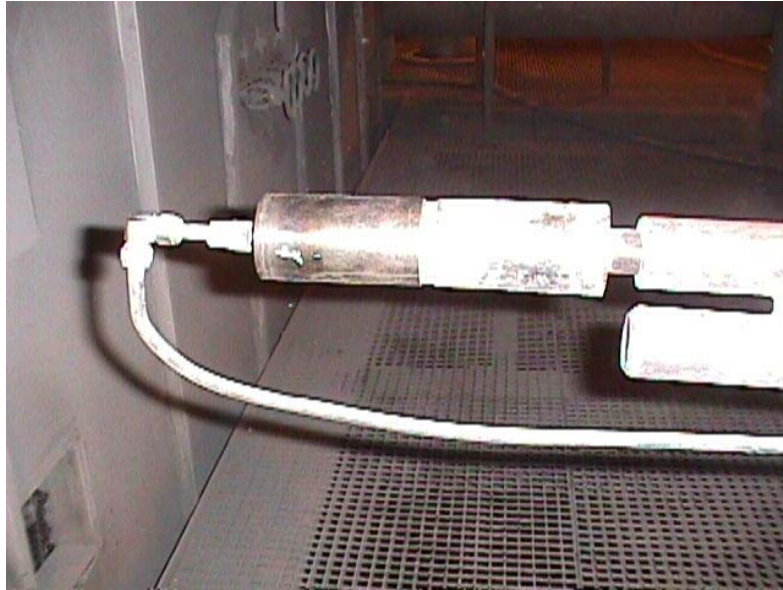
Figure C.4: Slag probe attached to top of the suction pyrometer. Cooling water is supplied to the front end of slag probe. Boiler wall is on the left of the photograph.
