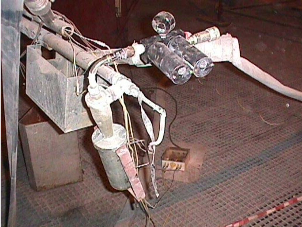
Figure C.6: The backend of the suction pyrometer illustrating the air-ejector (black) attached to the fly ash sample receiver.
