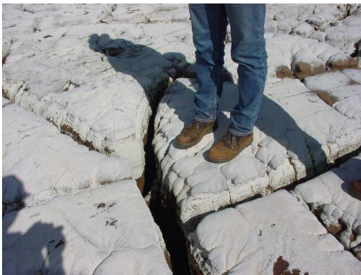
View of tailings basin. Note the consolidation cracking and the salt crystallisation.
