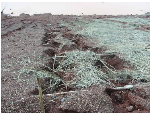
Erosion down the face of the starter wall. Note the timber used to retain mulch during germination.
