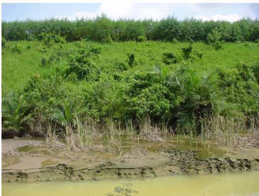
Sansu tailings facility – seepage from toe of revegetated impoundment wall.
