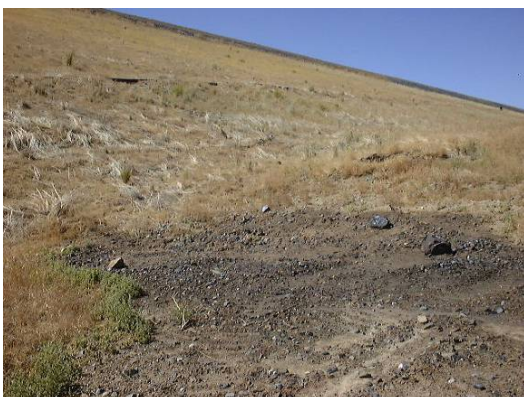
August 1999 – Outer face of the impoundment wall with vegetation.
