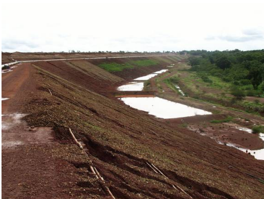
Subsequent erosion of section of the starter wall as a result of intensive rain.
