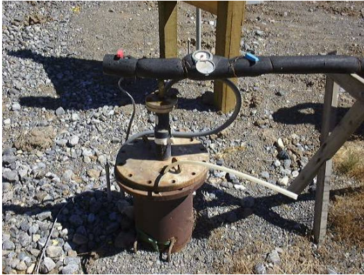
August 1999 – Abstraction well at tailings facility toe.
