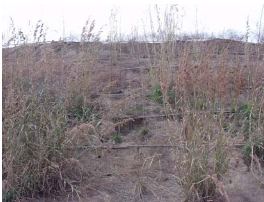
An eroded section of the cycloned material slope.
