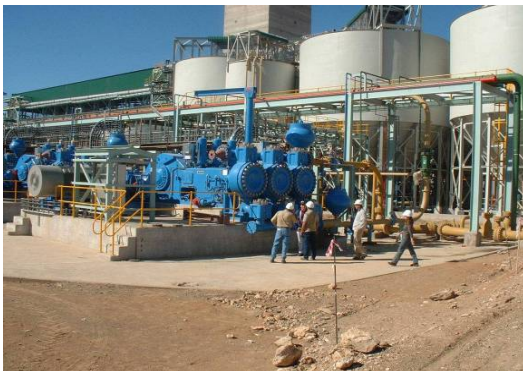
Positive displacement pumps for the delivery of thickened tailings to the tailings facility.
