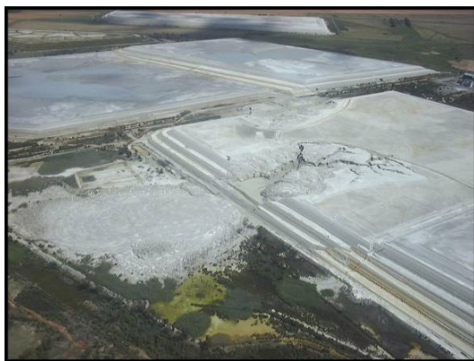
Figure 2.2.2: Slope failures of a ring dyke slimes dam in South Africa
