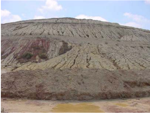
2001 – Erosion at external corner of tailings facility (Windy Corner).
