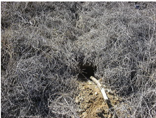
August 1999 – Localised seepage causing vegetation die-off.
