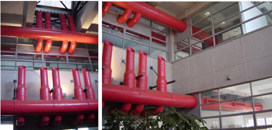
Figure 8 & 9 Images showing Exhaust system Author: 2005
