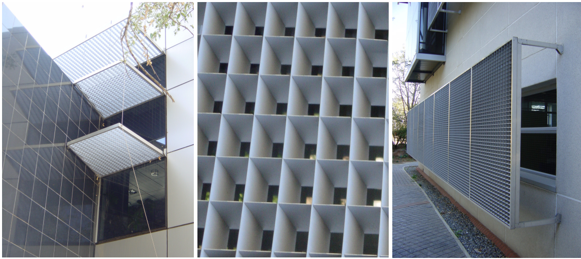
Figure 14, 15, & 16 Shading screens at BOTEC Headquarters
