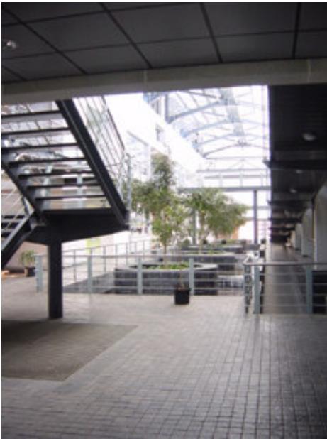
Figure 7 Image showing metal grating beneath staircase Author: 2005
