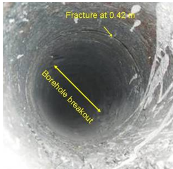
Figure G 41 Fracturing and slight borehole breakout observed in the Union P1 sidewall inspection borehole, drilled adjacent to the extensometer
