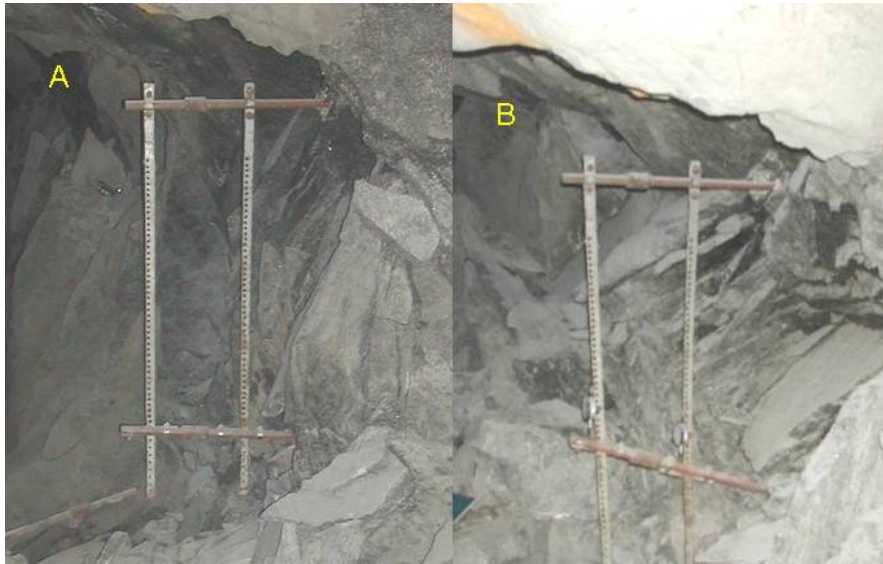
Figure E 3 Rotation of jumpers cemented into the centre of P2 near the top edge of the pillar and about 1 m vertically below. A = pillar failure, B = three months after pillar failure
