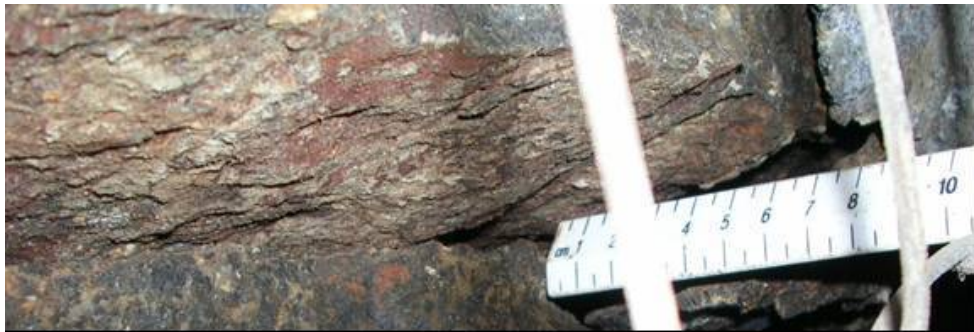
Figure E 60 Striations on the discontinuity surface, indicating a fault
