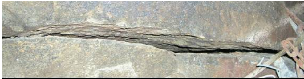
Figure E 59 Open discontinuity observed in the travelling way 1.3 m below Panel 8s
