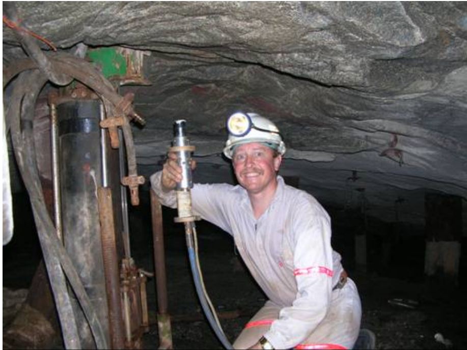
Figure B 6 Installation of a Doorstopper in a vertical borehole at the centre of a panel
