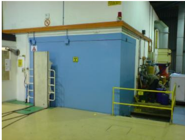
Figure 3.11: The sliding plug-door leading to the irradiation vault (coloured blue).
