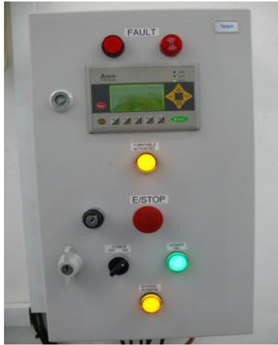
Figure 3.5: The main switchboard illustrating the main switch, warning lights for the rotating turntable, as well as “active source” and “fault” warnings for the entire control system.
