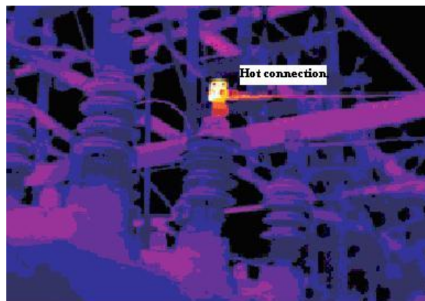
Figure 2.14: Thermal image of bushings in operation
