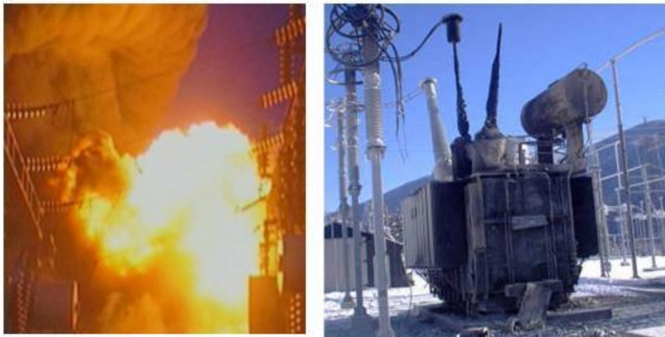
Figure 1.2: Destructive power of bushing failure
