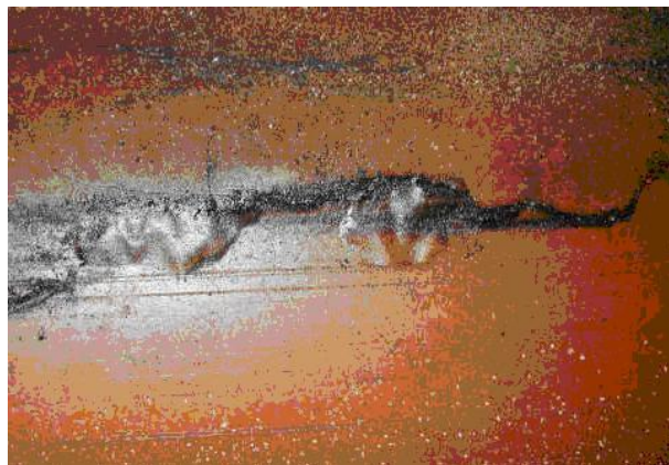
Figure 2.6: Carbonisation due to tracking on bushing paper insulation
