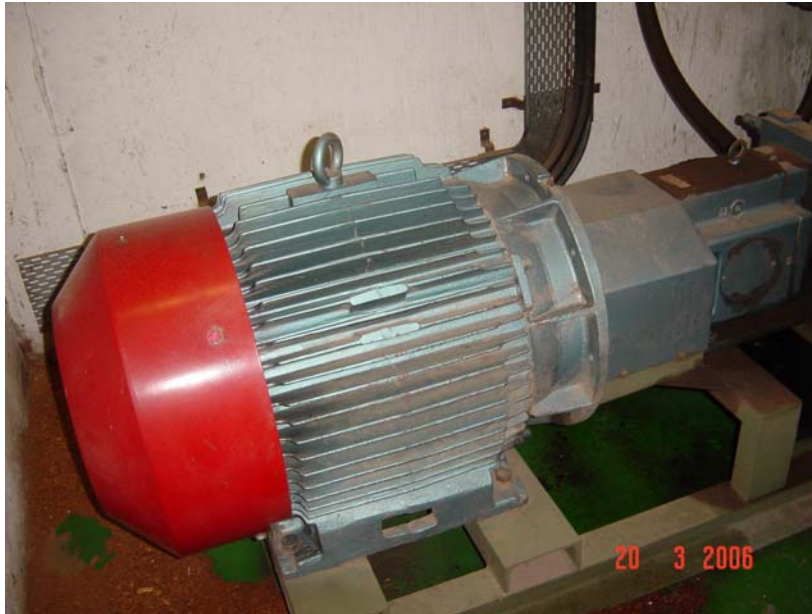
Figure 3.4 – Hydraulic Power Supply
