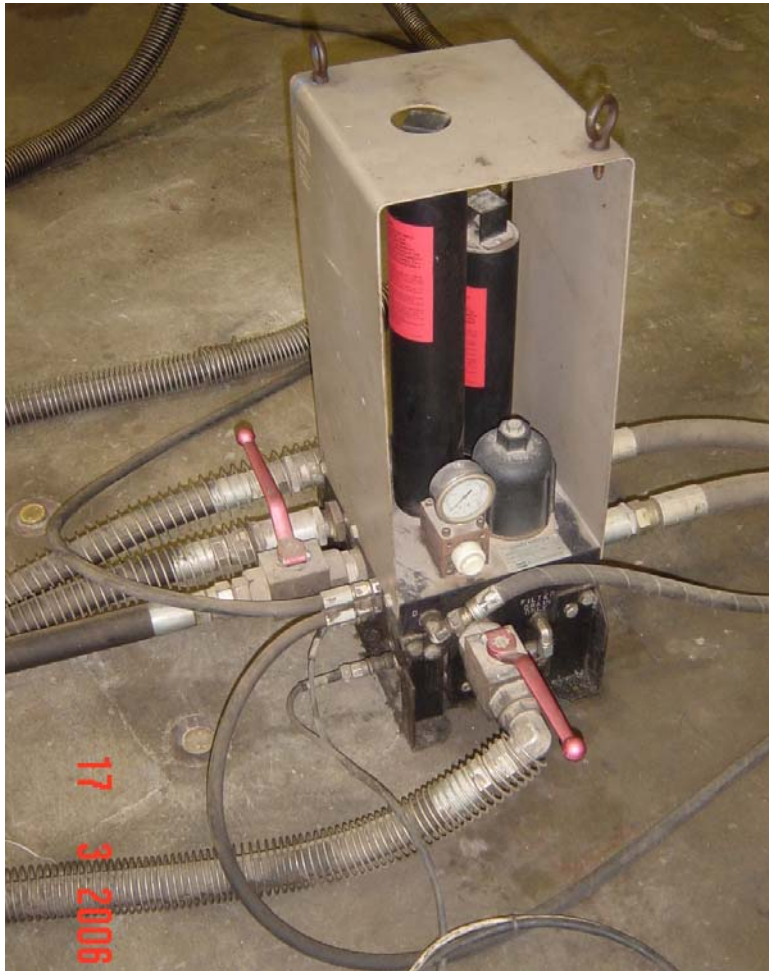
Figure 3.3 – Hydraulic Service Manifold
