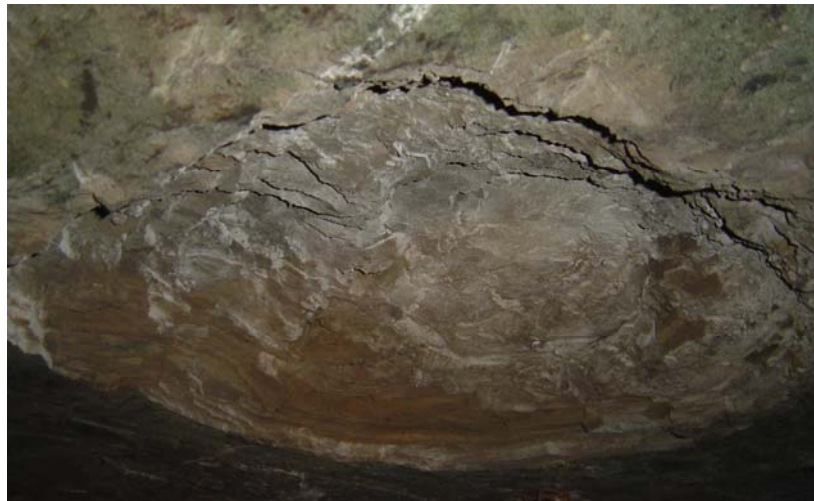
Figure 3.21: Fall of muddy roof
