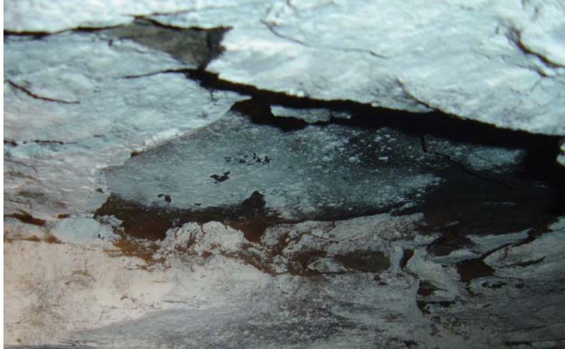
Figure 3.22: Occurrence of guttering in combination with slabbing was common in muddy roof
