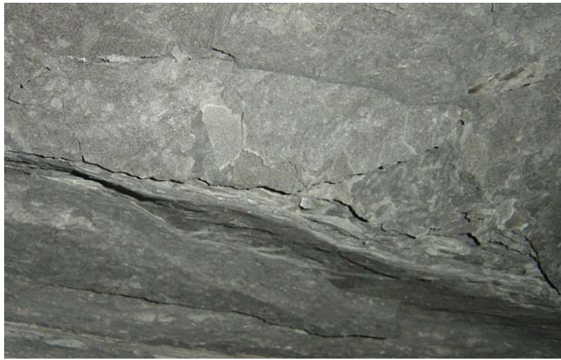
Figure 3.5: Photograph showing a fractured roof which on scaling results in a gutter
