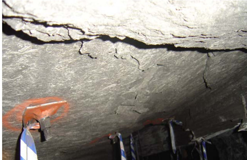
Figure 3.14: Occurrence of roof guttering along roof bolts
