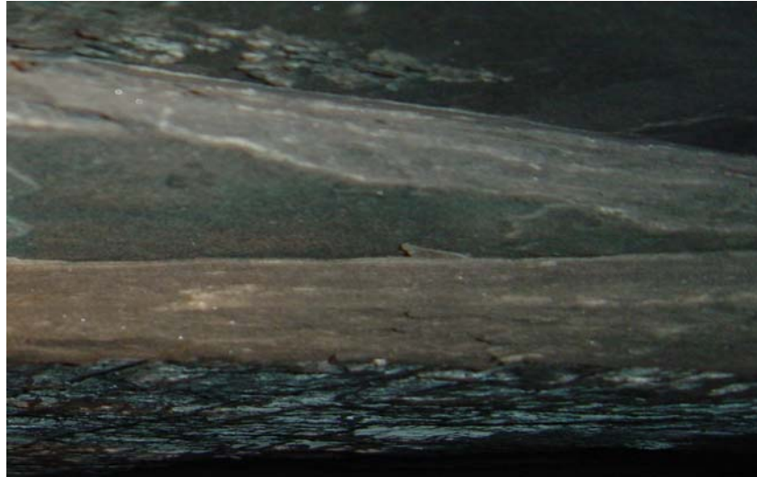
Figure 3.19: Photograph showing roof slabbing initiated by roof guttering
