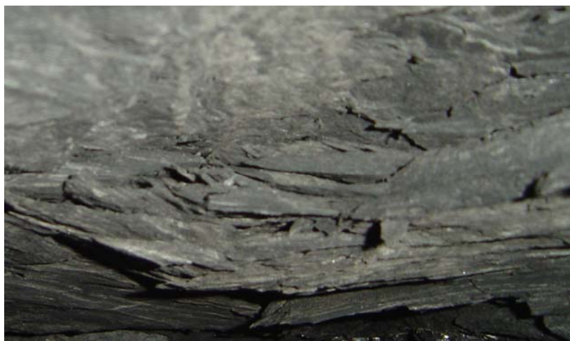
Figure 3.10: Photograph showing stress induced fracturing ahead of a gutter. The roof gutter occurred towards the centre of a roadway
