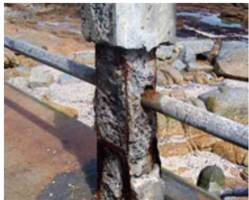
Figure 1. Reinforcement corrosion remains the most significant threats to the durability of reinforced concrete structures.
