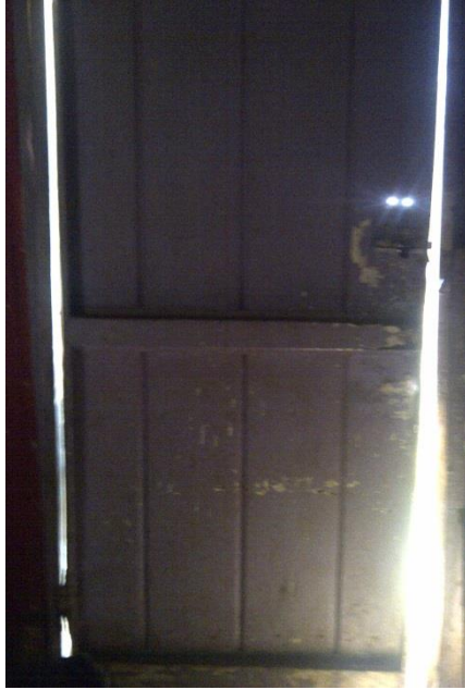
Figure 10: Poorly installed door
