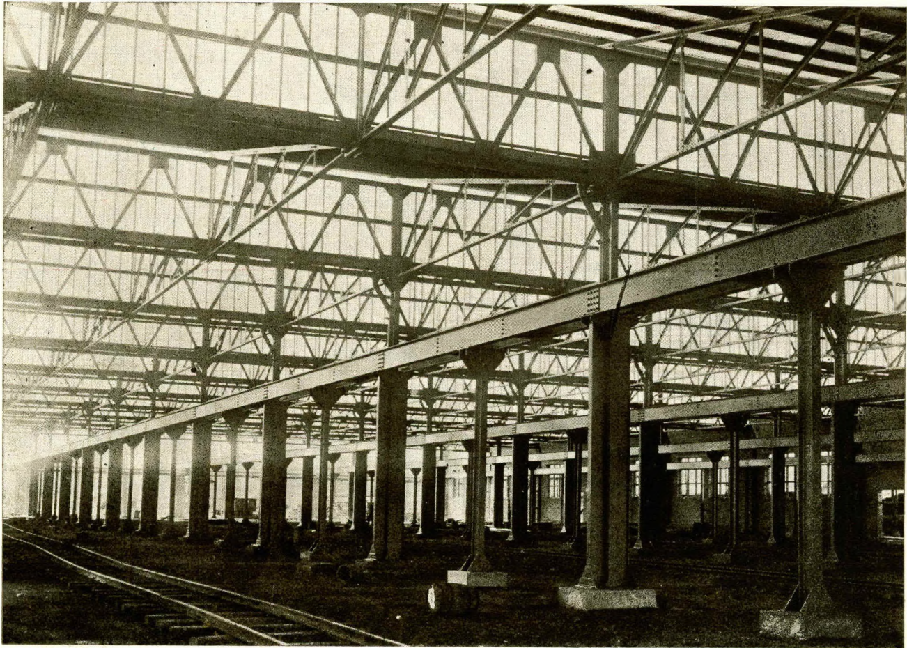
Internal View New Wagon Shops, S.A.R., Maritzburg. Total weight of structural steelwork nearly 1,000 tons. Supplied and erected by us complete.
