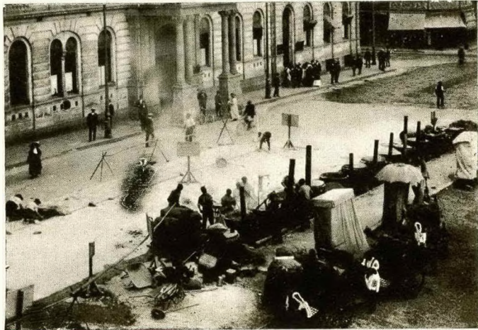
Photo of Asphalt Road being laid by Jenkins & Co., outside G.P.O., Johannesburg
