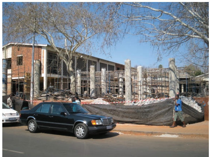
FIGURE 25: 2009: the Yeoville Recreation Centre in the process of being re-modelled. This is arguably the least successful of the JDA projects. There are some design problems and the quality of work is inconsistent and, in some cases, very poor. However, far worse is the state of the building today – only four years since the upgrade, it is in a shocking state. It is an indictment of the Department of Sport and Recreation that they have allowed a building in which millions was invested to deteriorate to the extent that it has.
