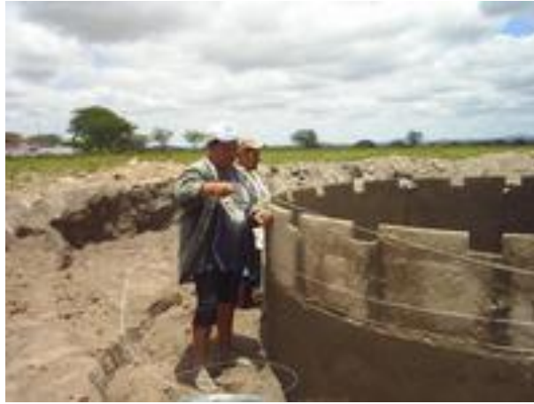
Fig. 15. A Brazilian woman using her masonry skills to construct a tank for income. Photo: GWA, 2008. Source: Nogueira, 2008
