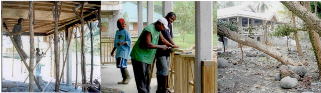
Figure 8.9. Construction of the Rosalie Bay ocean-view cottages, which are the subject of the “value chain” analysis
