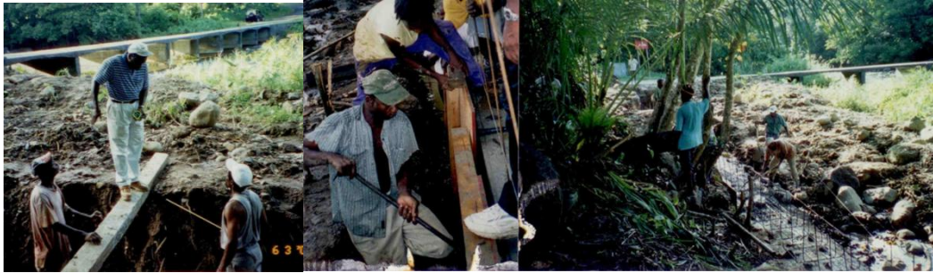
Figure 8.4. Early construction images from 2002 showing the hand digging and pouring of foundations at Rosalie Bay
