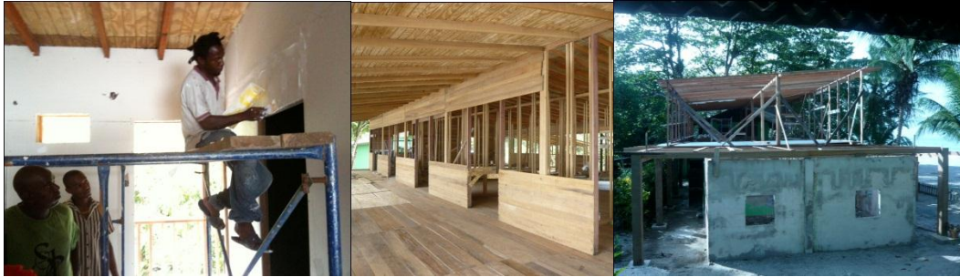
Figure 8.12. Construction of the new second story extension of Mt. Plaisir, which is the subject of the “value chain” analysis Source: Photographs by Piero Guerrini
