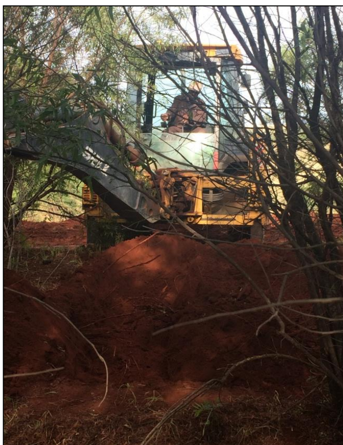
Figure 3.5. TLB trying to dig a soil pit through two outer trees of a plot; one of the difficulties the TLB encountered whilst digging soil pits.
